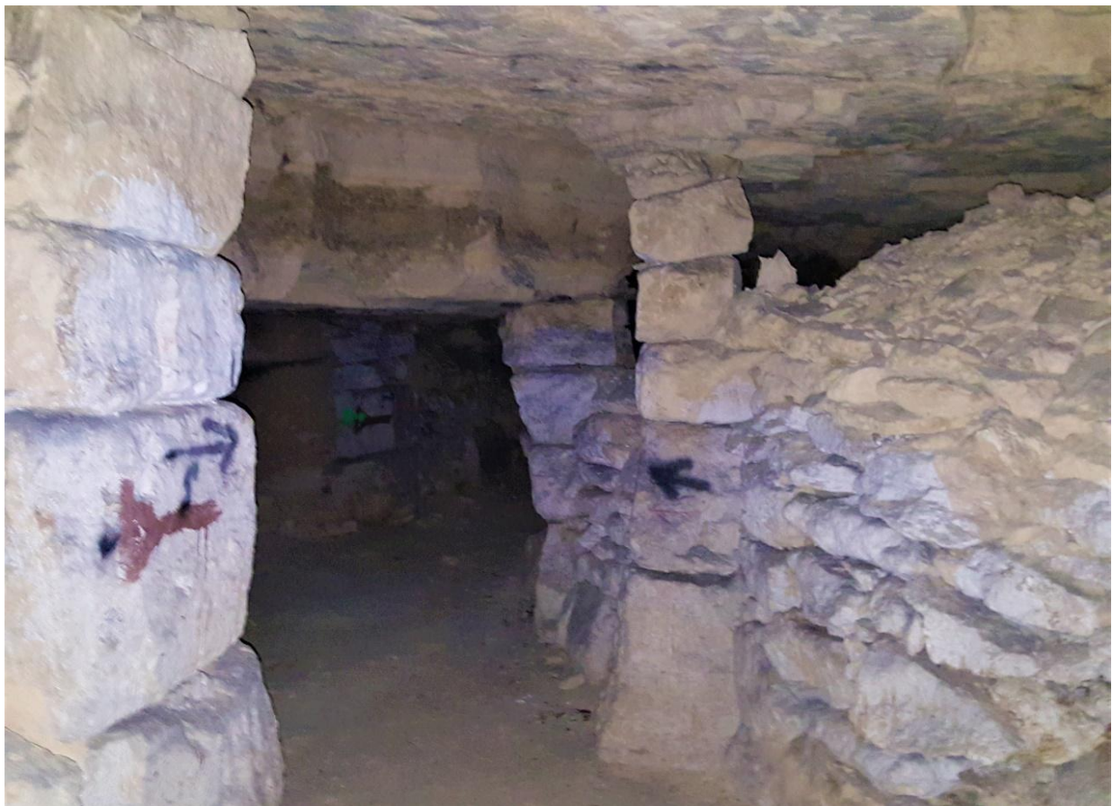
Stone-walling and back-filling extraction in underground quarry at Bazemont (Yvelines) © J.-P. Gély
